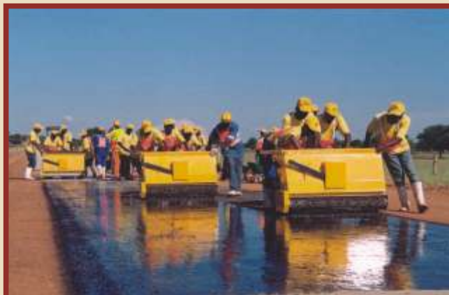
The aggregate is loaded into the "Chippy" by wheelbarrows and the "Chippy" guided along the length of the road in accordance with the manufactures instructions.
